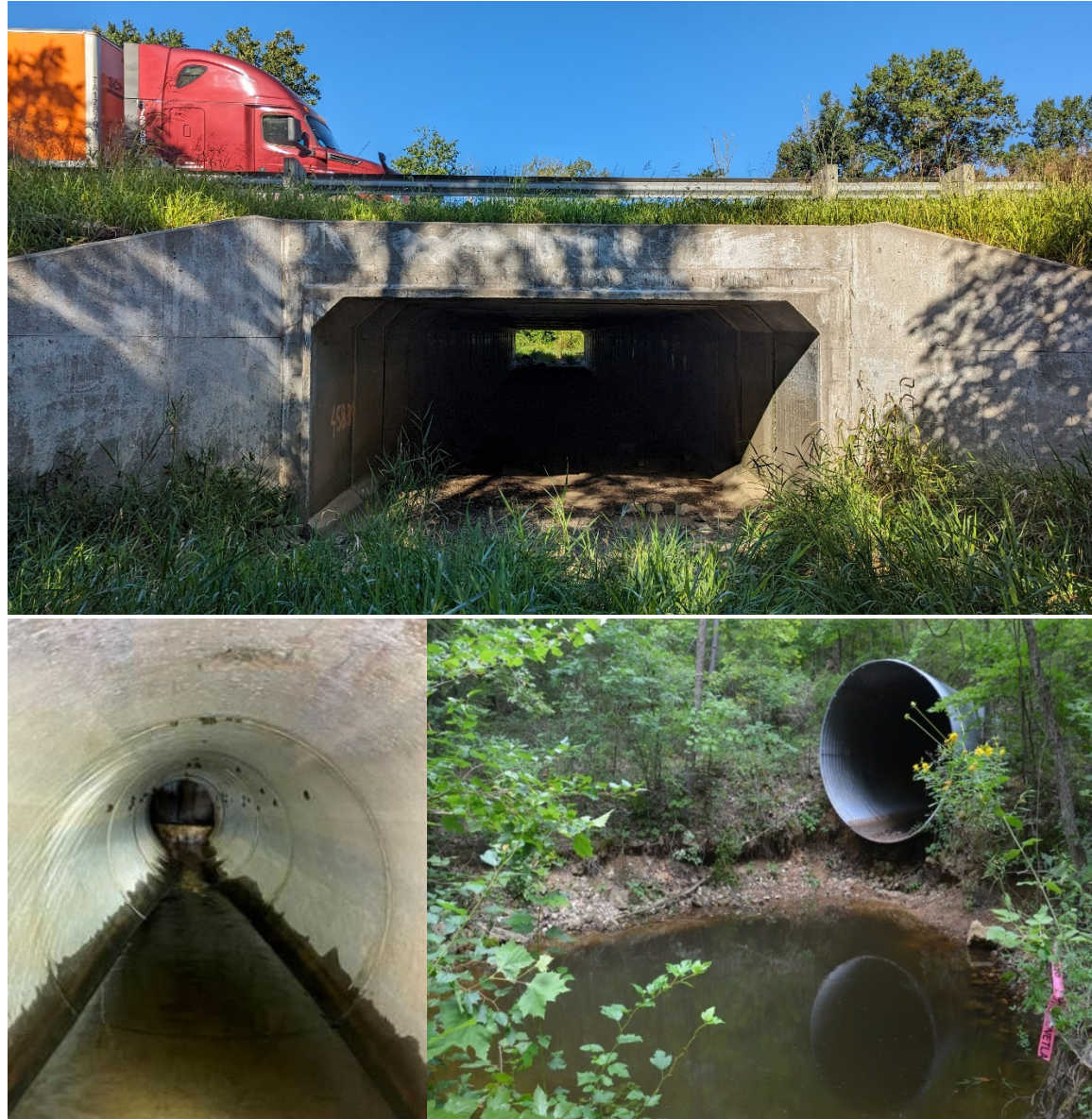
FIGURE 8. Representative culvert structures of various types, including a box culvert in Indiana (top; photo by USFWS); a round, concrete pipe culvert design in Georgia (bottom left; photo provided by Georgia Department of Natural Resources); and a corrugated metal pipe culvert design in Missouri (bottom right; photo provided by L. Droppelman).
