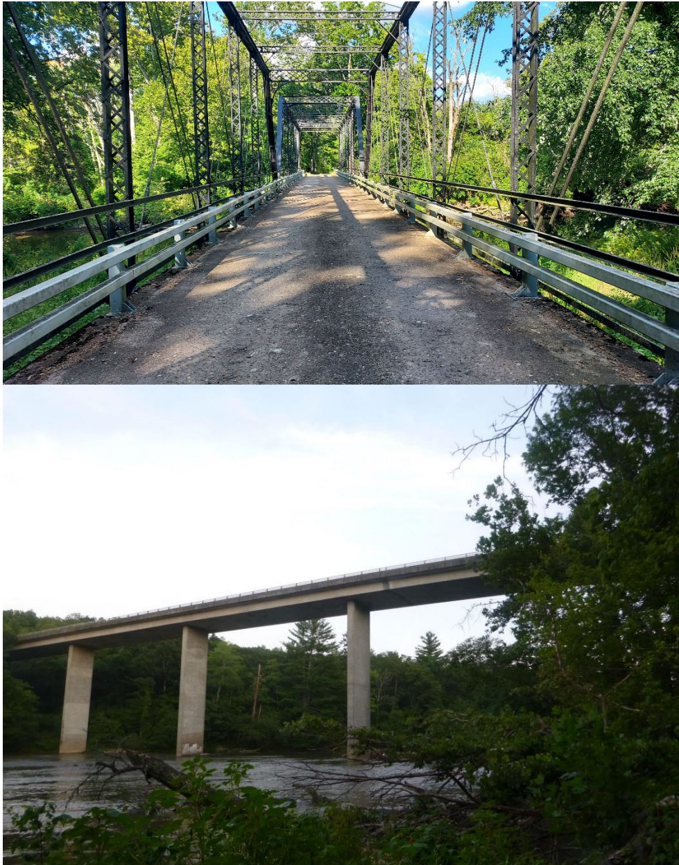
FIGURE 9. Representative bridges with documented bat use, including a bridge with metal struts in Indiana (top; photo provided by Indiana Department of Transportation) and a concrete bridge in North Carolina (bottom; photo provided by North Carolina Wildlife Resources Commission).
